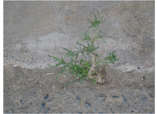
Stinkwort emerging through asphalt on industrial site
